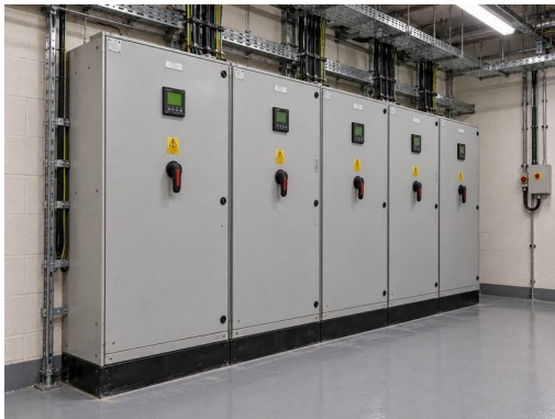
Photo 9: Main LV switchgear, electrical service room
