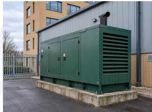
Photo 10: Standby generator, rear service yard
