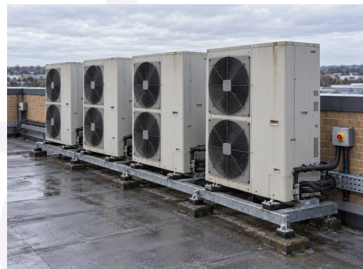
Photo 6: VRF condensing units, roof plant platform
