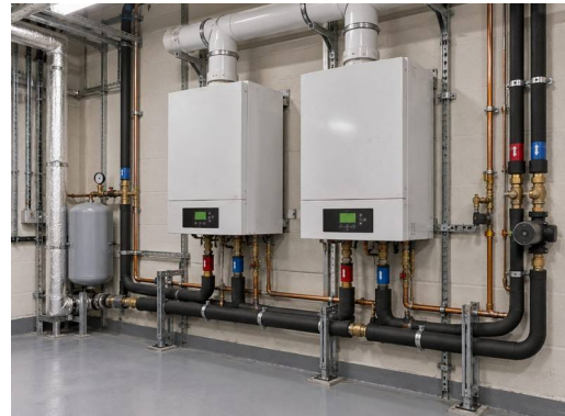
Photo 2: Gas condensing boilers, main plant room
