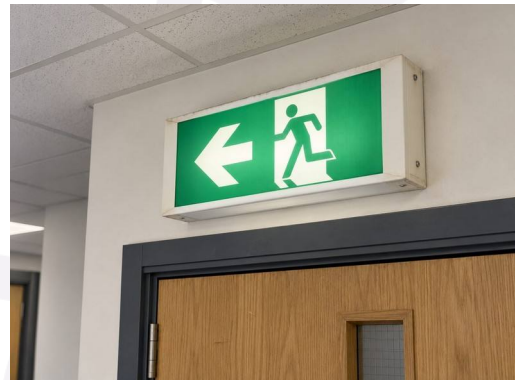
Photo 12: Exit sign, ground floor corridor
