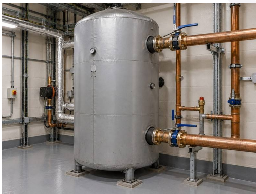
Photo 3: Calorifier, main plant room
