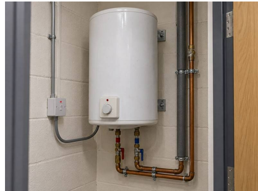
Photo 8: Electric water heater, office wing kitchenette
