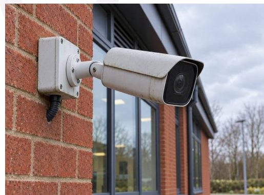
Photo 14: External CCTV camera, office wing
