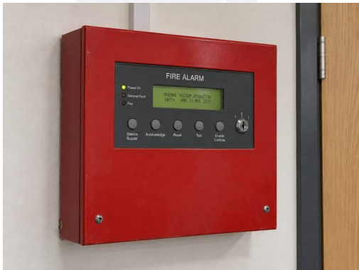
Photo 11: Fire alarm panel, ground floor entrance
