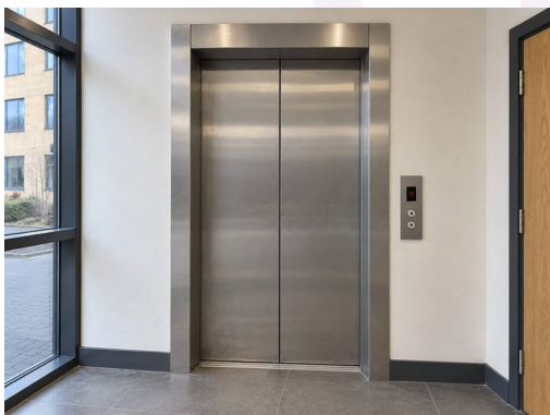
Photo 13: Passenger lift, ground floor lobby
