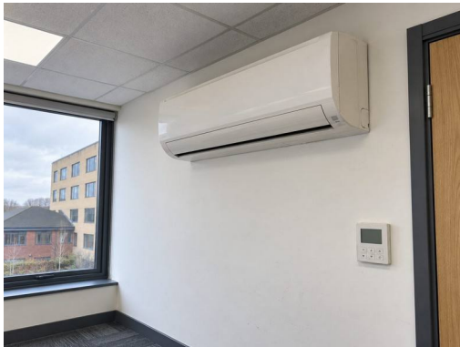
Photo 7: Split unit, office wing meeting room
