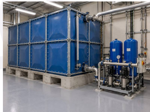
Photo 4: Cold water storage tank and booster set
