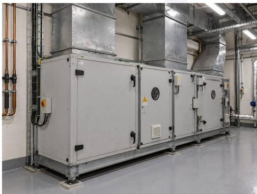
Photo 5: Air handling unit, main plant room
