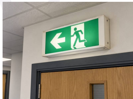
Photo 14: Exit sign, ground floor corridor
