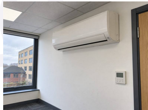
Photo 17: Split air conditioning unit, meeting room
