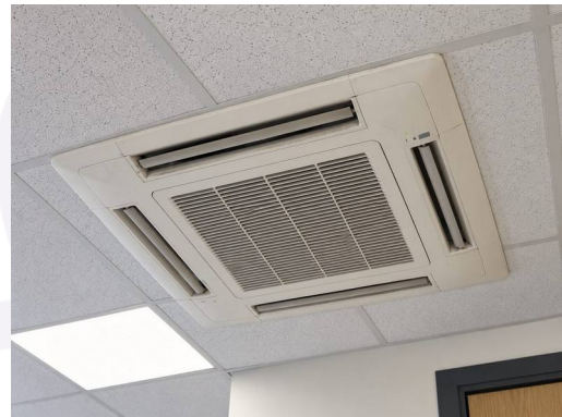
Photo 10: VRF ceiling cassette, typical office floor
