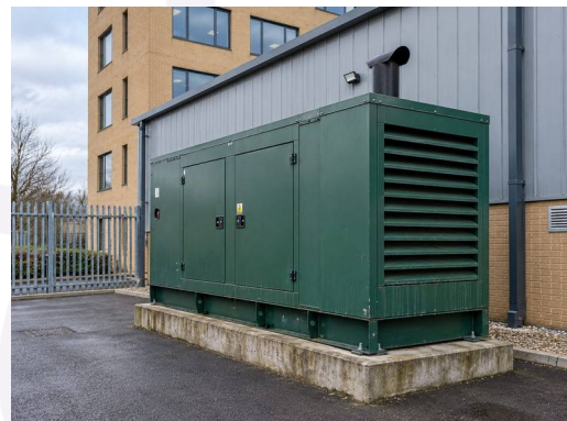
Photo 24: Standby generator, rear service yard
