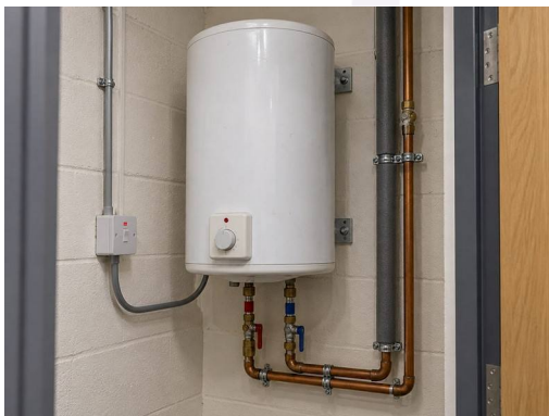
Photo 18: Electric water heater, kitchenette
