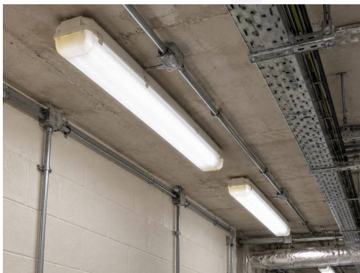
Photo 23: LED batten fittings, service corridor
