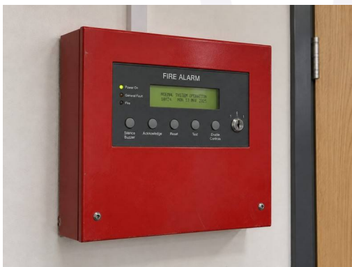
Photo 13: Fire alarm panel, ground floor entrance
