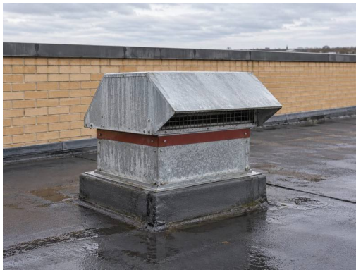
Photo 9: WC extract cowl, main roof
