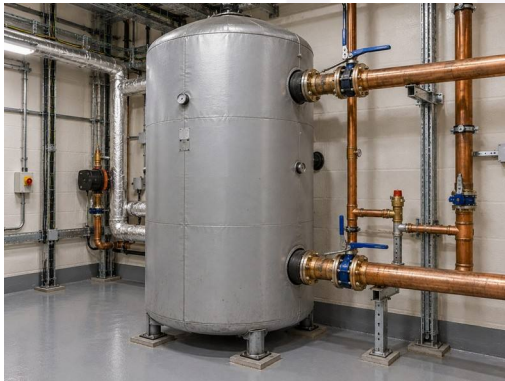
Photo 3: Calorifier, main plant room
