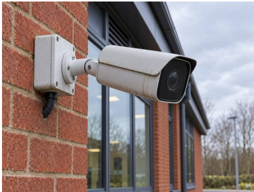
Photo 20: External CCTV camera
