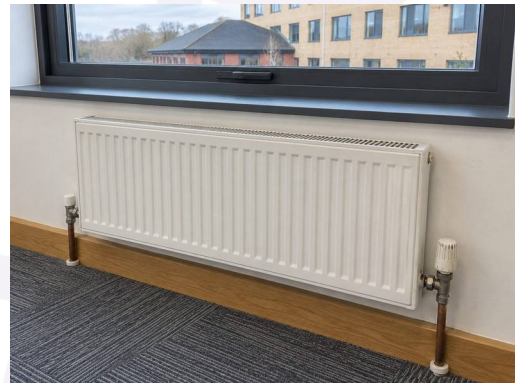
Photo 12: Perimeter panel radiator, office floor
