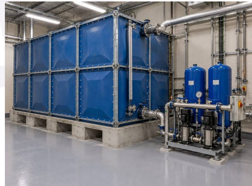
Photo 4: Cold water storage tank and booster set
