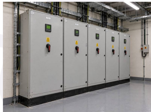
Photo 6: Main LV switchgear, electrical service room
