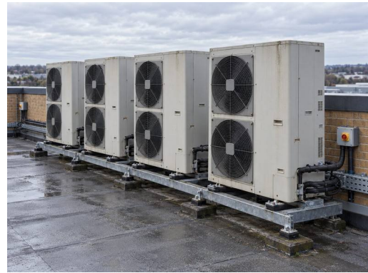
Photo 8: VRF condensing units, roof plant platform
