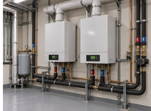
Photo 2: Gas condensing boilers, main plant room
