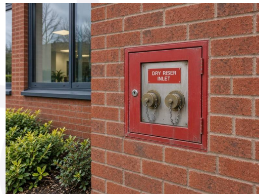
Photo 19: Dry riser inlet, front elevation
