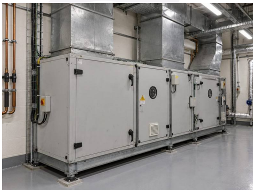
Photo 5: Air handling unit, main plant room
