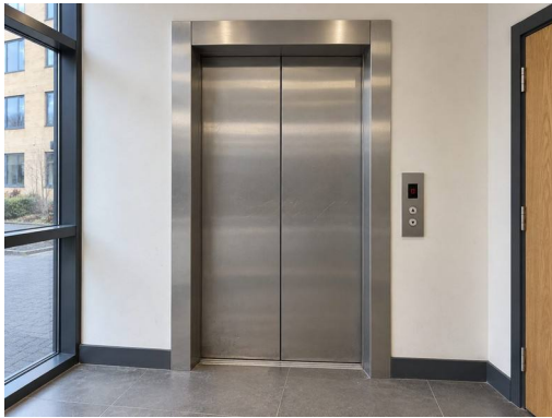
Photo 15: Passenger lift, ground floor lobby
