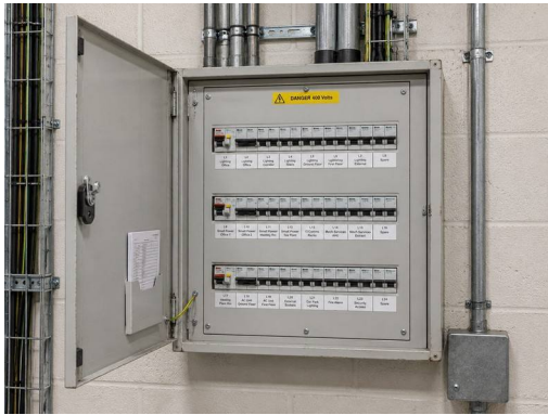
Photo 7: Typical floor distribution board
