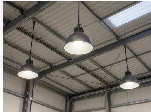
Photo 22: LED high bay lighting
